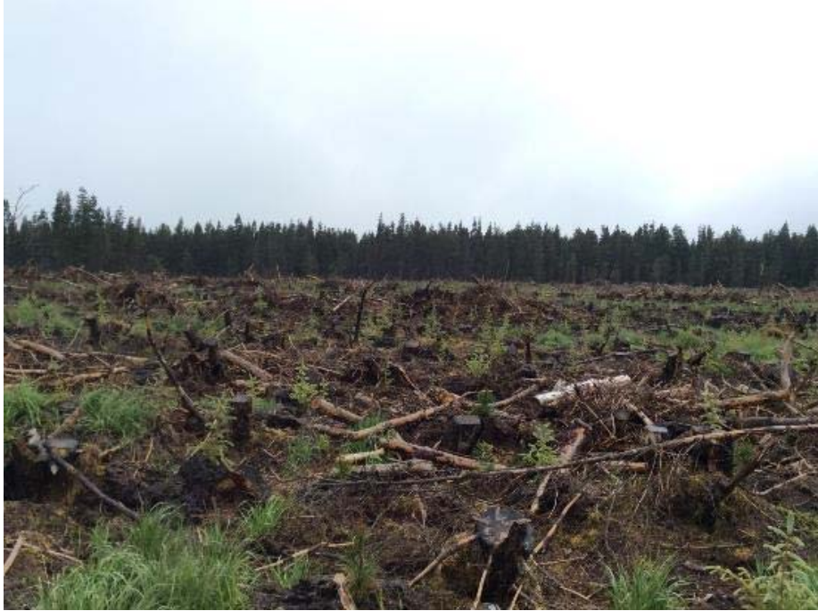
Plate 1-43: Proposed hardstand for T3 and vicinity of turbine base looking south west.
